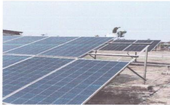
Fig. 1a. Solar Panel
