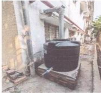
Fig. 7. Rain Water Storage Tank
