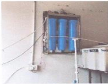
Fig. 8. Part of the RO unit
