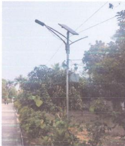
Fig. 1b. Solar Street Light
